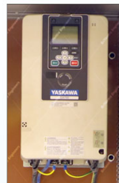
Digital VFD with noise filters (Variable Frequency Drive)
